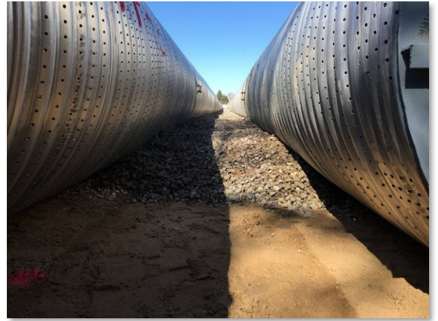
(Above left) The infiltration gallery consists of 25 rows of interconnected pipe - over 1.42 miles of it.
